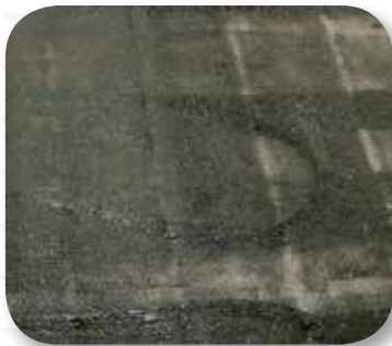
X Light Coverage Will cause lack of adhesion.
